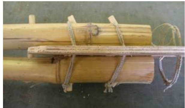
Figure 9. View of a collapsed joint.
